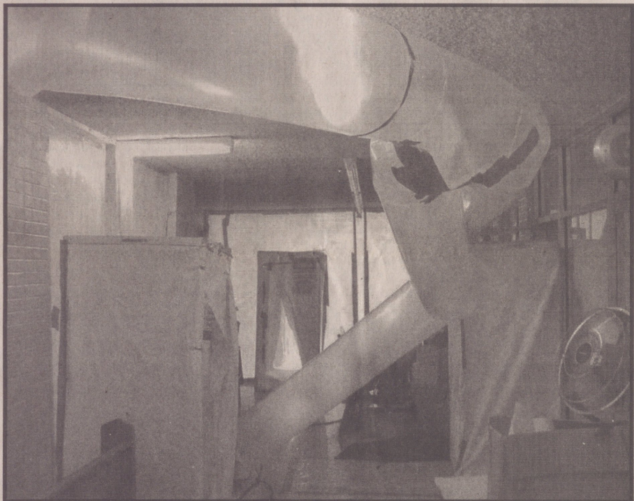
The Senior Hallway during the summer. These tubes are to contain the asbestos the workers had to expose during their remodeling.
