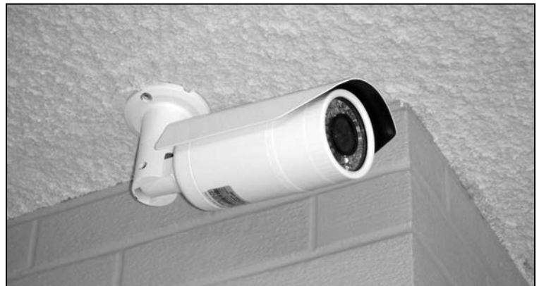
Many new security cameras were added to both the interior and exterior of the school as part of the new security enhancements made this year.
